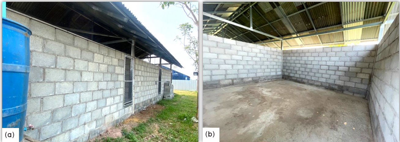
Figure 7 Equipment and materials storing building and worker's changing room; (a) Outside building and (b) Inside building
